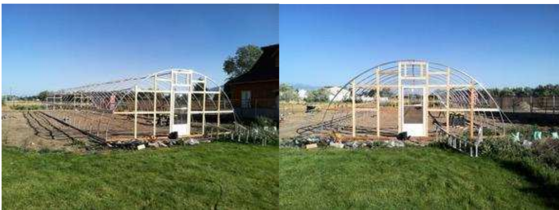
Figure 23 – Hightunnel with framing. Note opening for a bay door on back side (Right)
